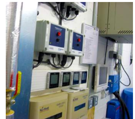
^ Site Photo: MVHR unit, Haywood Green Farm
